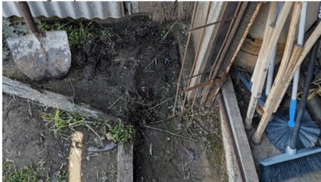
A critical issue is keeping silt out of the drain after clearing it. Grates help but replacing the earth with roadbase is probably the best start
