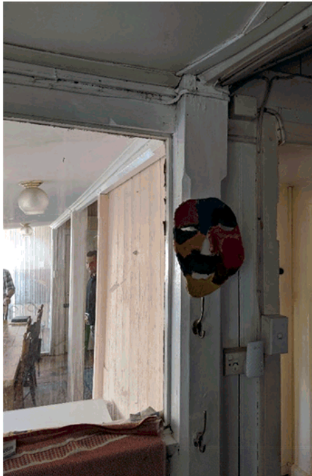
3. Original corner verandah post and chamfered lintel beam to be retained for reuse
