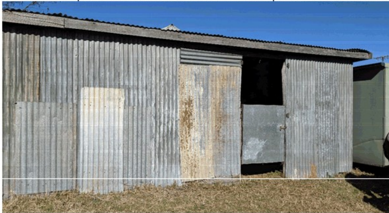
Barn stable doors to be reinstated Perimeter gravel roadbase 1200mm wide perimeter Barge roll flashing to be fitted to conceal the edge shown above Timber fascia to be painted as per the Cell notes
