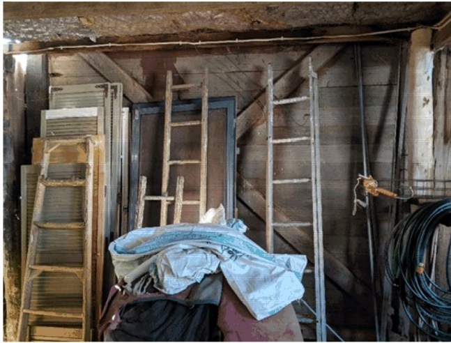
The side of the cell building exposed inside the stable. Clearing these items away from this wall would look best to stack them against a less important wall and ensure the timber can be inspected – termites remain a big threat.
