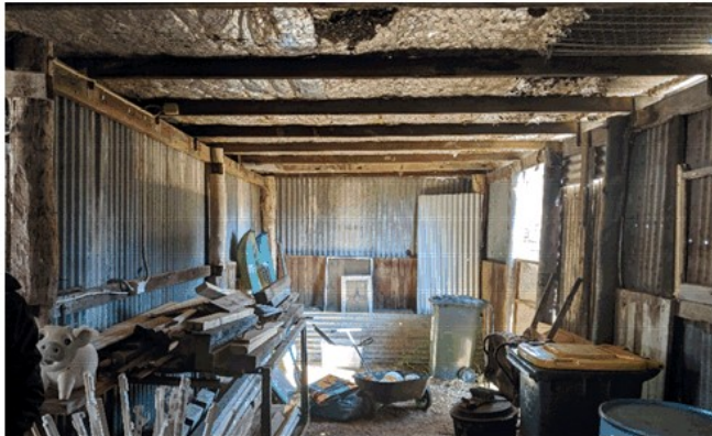
Long view of the stable: the exposed sisalation foil is not a good look in a heritage building. Options: Line the underside of the rafters with recycled galvanised iron sheet
