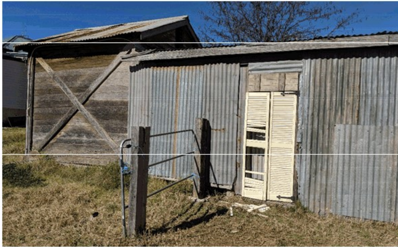
The junction with the stable wall works well with a simple working flashing. The two fence posts above to be restored and developed further into the fence line and gates
