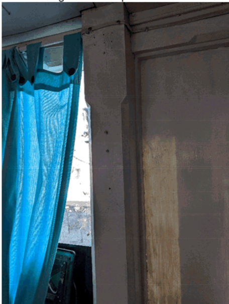
2. Original timber chamfered verandah post and lintel to be reused in the new verandah
