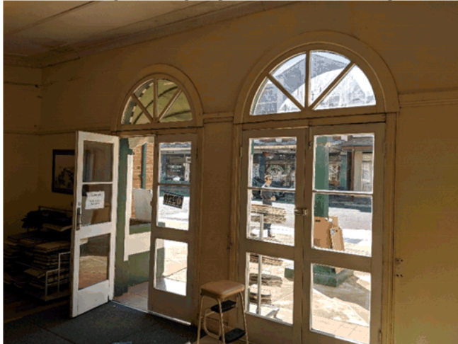
View from the lobby entry space, noting the importance of the doors and fanlights. Note the surrounds, picture rail and cornice The ceiling includes moulding details worthy of restoration. Lights for the ceiling could be similar to the following
