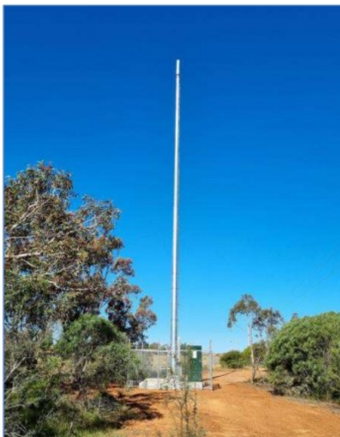
Figure 5 – Similar Telstra small cell facility.
