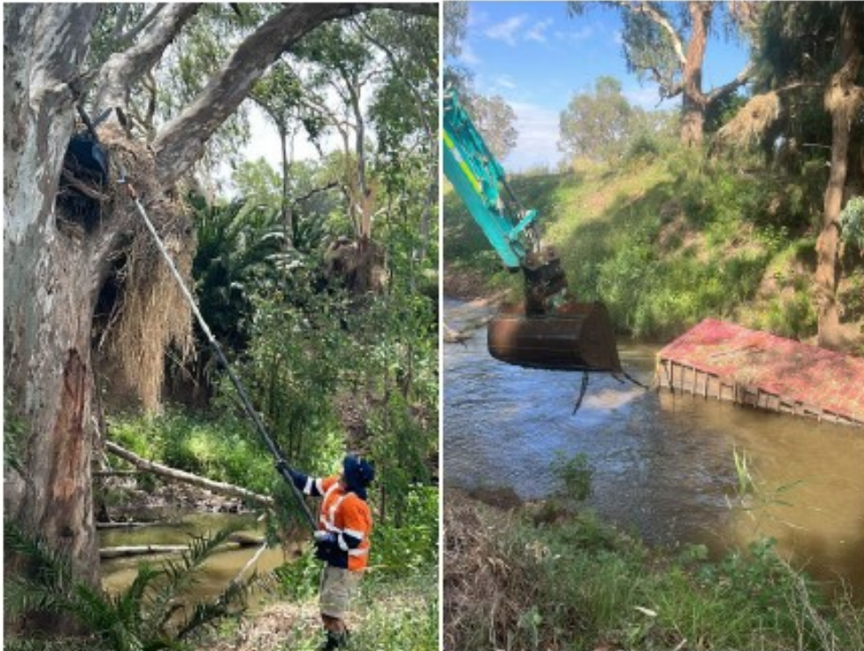
Flood debris in Eugowra.
