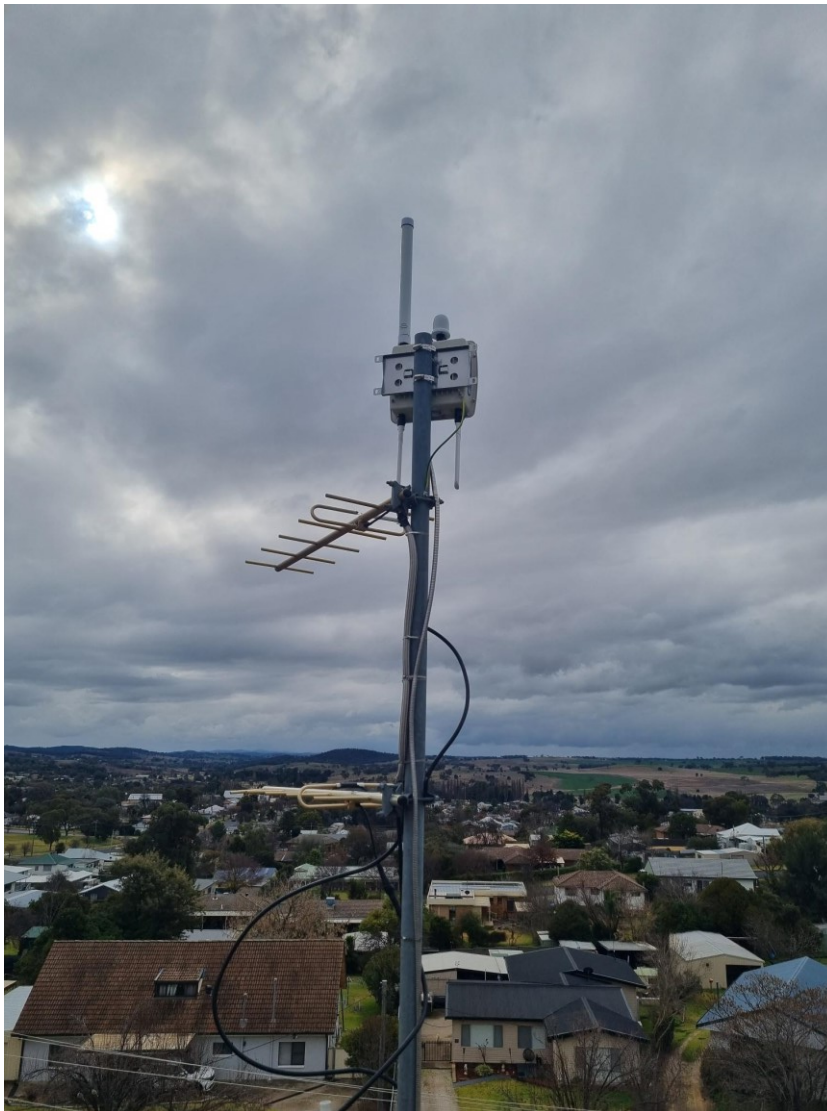
LoRaWAN Gateway mounted on the Molong Water Treatment Plant (top device)
