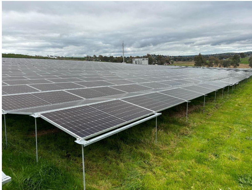
Photo 1. Example solar array powerplant
