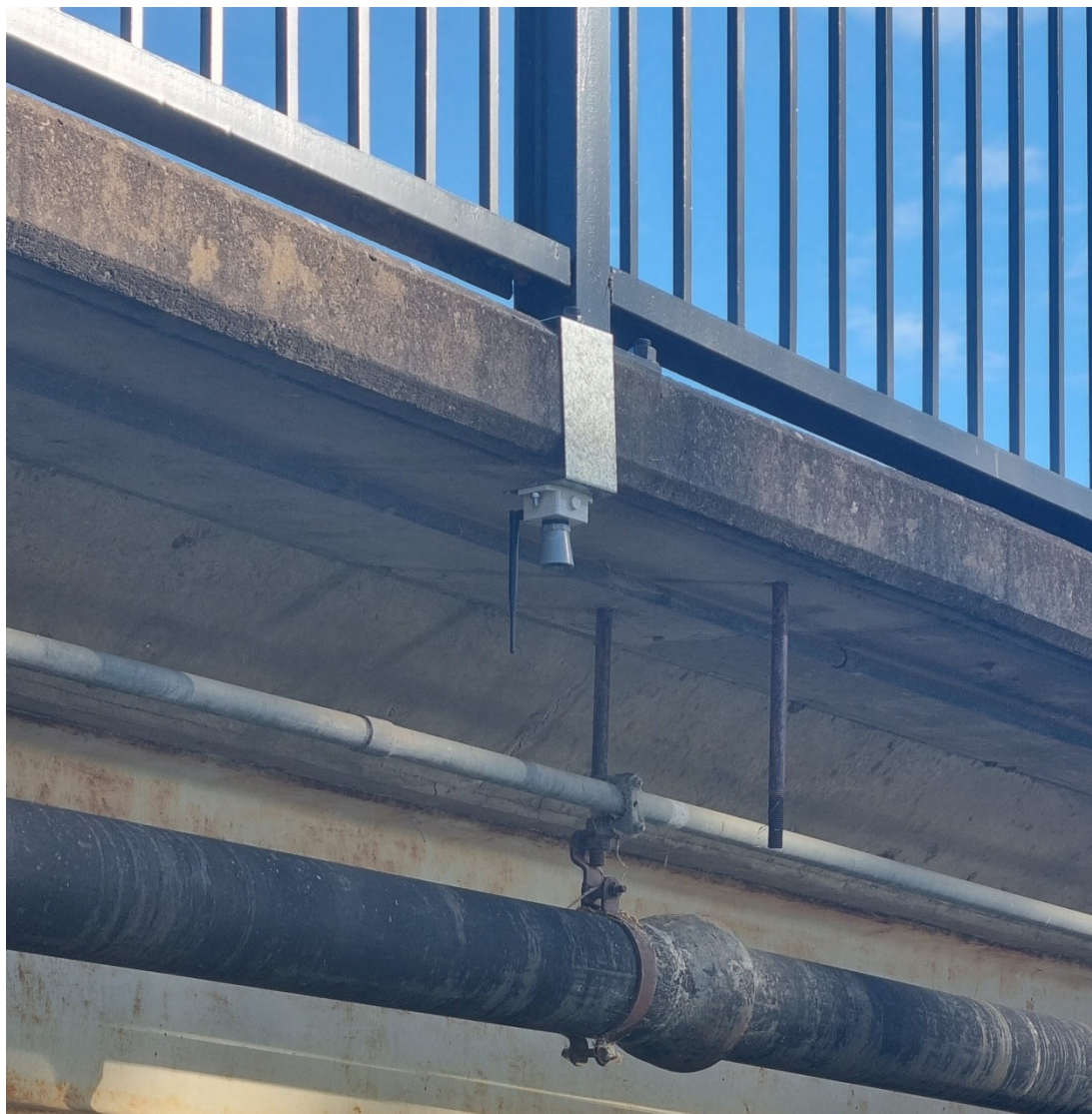
Sensor mounted on bridge
