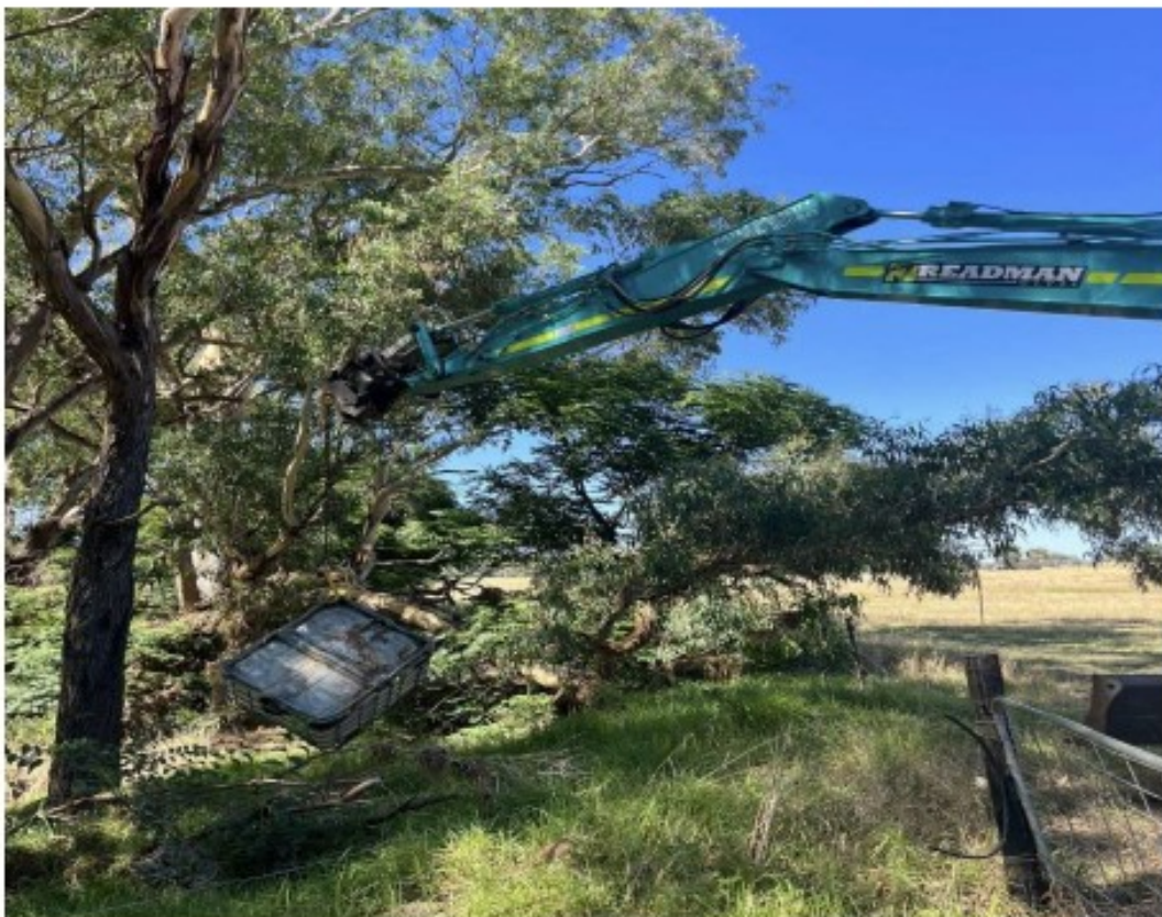
Flood debris removal in Eugowra.
