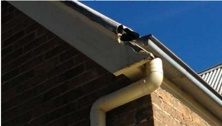
Figure 21 Missing spear point and flashing and eroded barge board end
