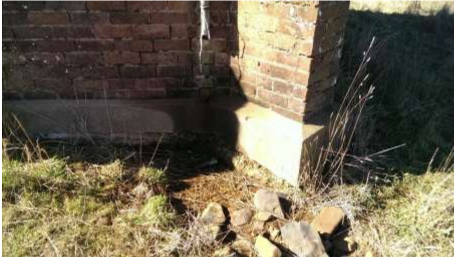
Figure 15 Water damage and missing downpipe
