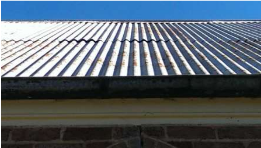
Figure 10 While the roof sheeting looks fine, many fixings are raised and the end laps have opened allowing wind blown rain to enter the roof space.
