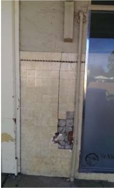
Damage to the Vinnies wall on both the tiles and the brickwork, noting the vertical movement.
