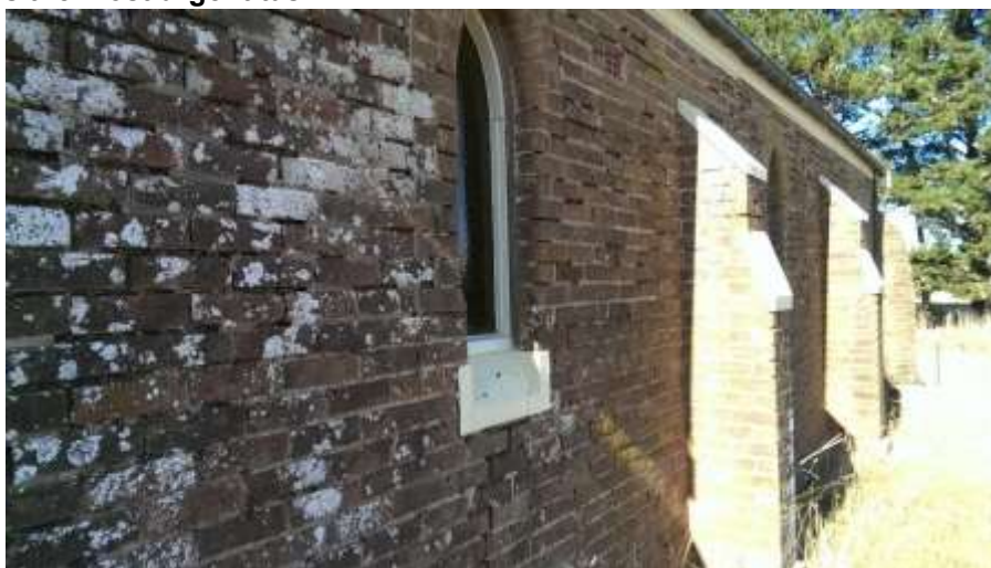
Figure 17 Side elevation showing the missing pointing caused by the leaking guttering.
