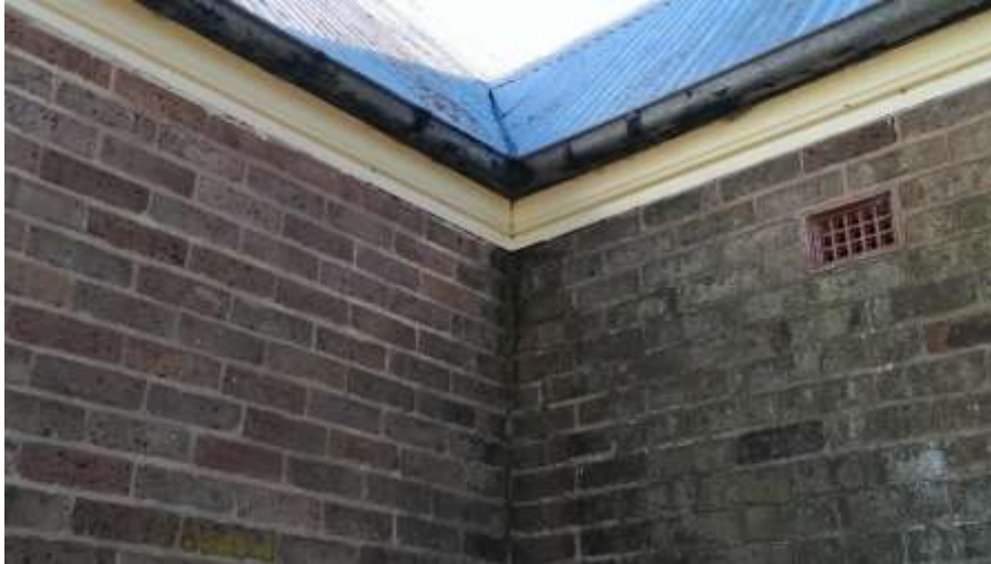
Figure 7 The internal corner is not draining to the downpipe and overflows are damaging the brickwork and foundation. Refer the following image.
