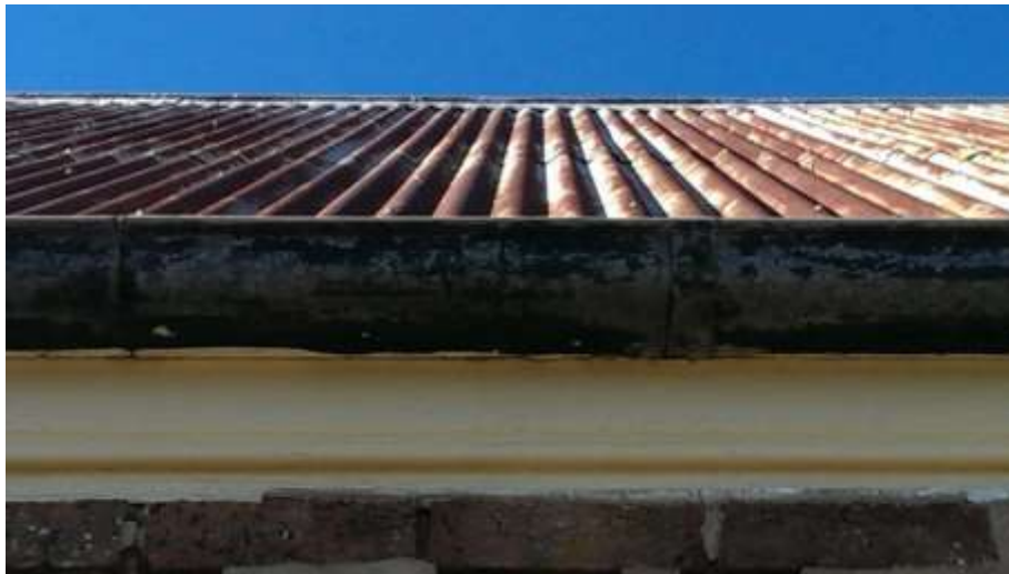
Figure 16 Note rust damage and raised fixings. The guttering is completely eroded through and replacement galvanised steel guttering and downpipes are required. This is the most urgent task.
