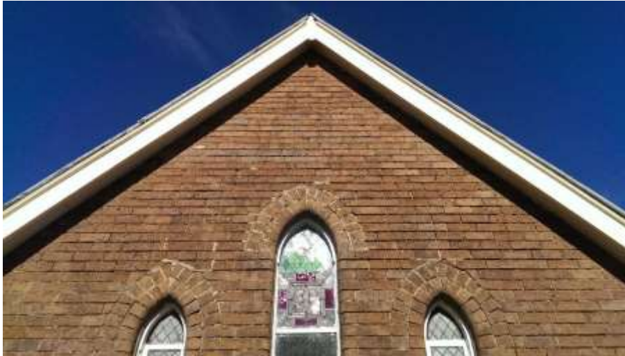
Figure 18 The missing cross and general view of the brickwork and missing pointing.
