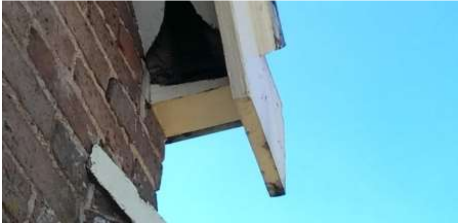
Figure 12 Damaged timber at the eave and barge board junction
