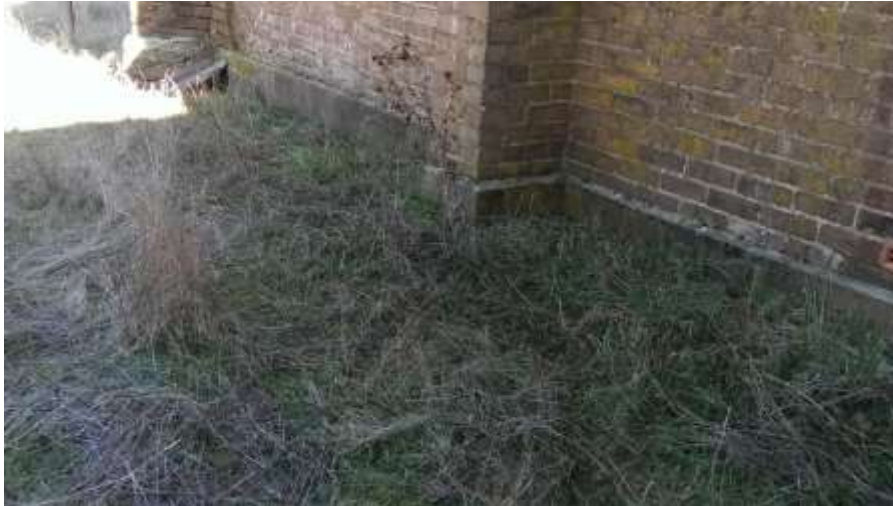
Figure 4 Typical view of the perimeter where weed growth is against the building promoting rising salt damp
